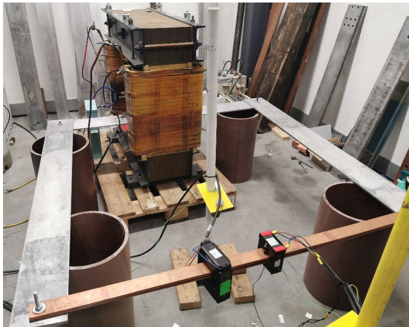
e) 600/5A CT Photograph no. B26-20-AA-05E/04 Temperature-rise test
