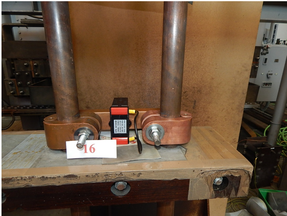
f) 1000/5A CT Photograph no. B26-20-AA-06E/05 Short-time current tests
