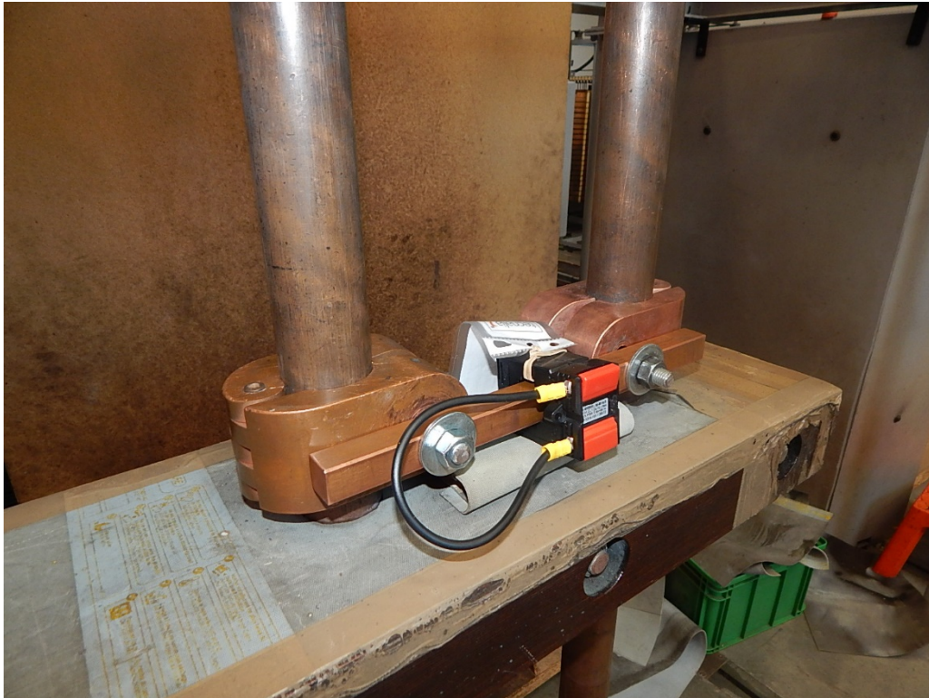
d) 400/5A CT Photograph no. B26-20-AA-04E/05 Short-time current tests
