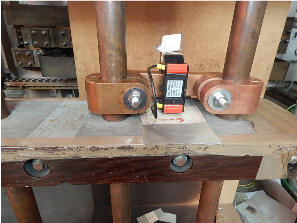
g) 1600/5A CT Photograph no. B26-20-AA-07E/05 Short-time current tests
