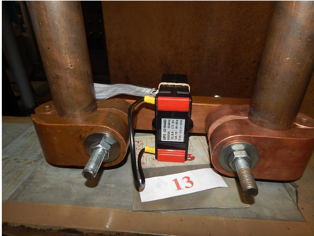
e) 600/5A CT Photograph no. B26-20-AA-05E/05 Short-time current tests
