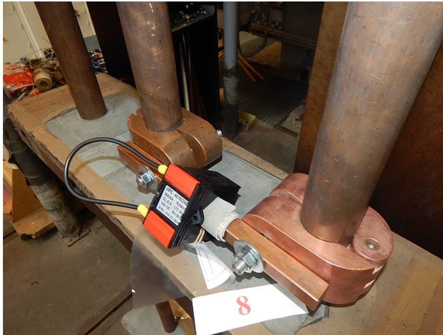
c) 300/5A CT Photograph no. B26-20-AA-03E/05 Short-time current tests
