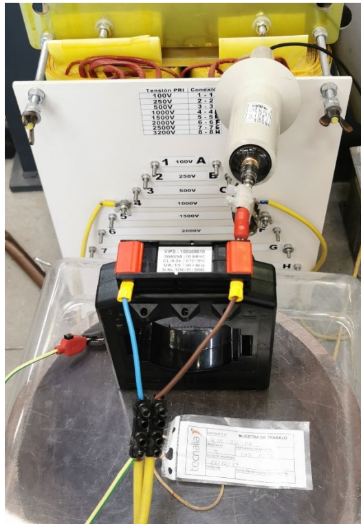
i) 3000/5A CT Photograph no. B26-20-AA-09E/03 Inter-turn overvoltage test
